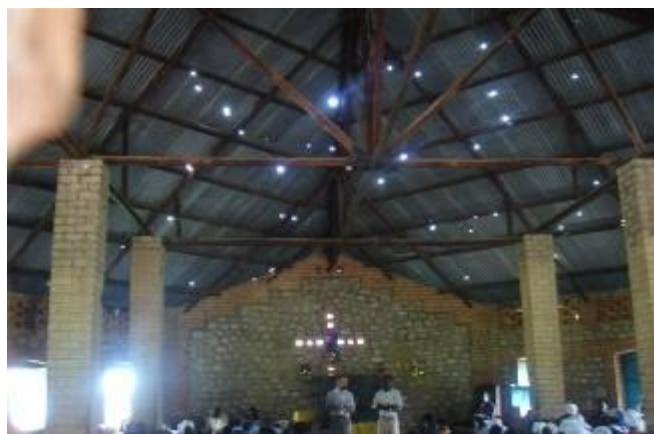
The Cathedral Church of Lazarus, holes in roof are from shrapnel
